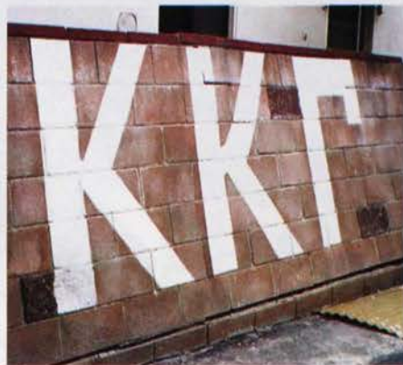
Wall cracks and other structural damage are prevalent at the Epsilon Xi house.
